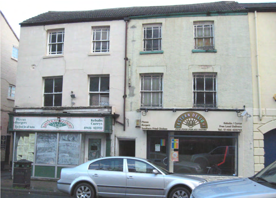
Plate 65: A pair of prominent unlisted properties on High Street which are failing in terms of their condition.
