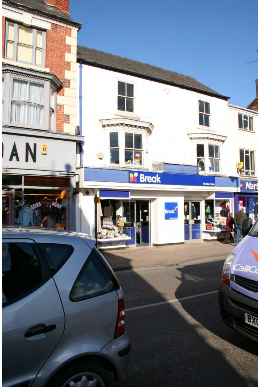
Plate 32: Unused upper floors and windows blighted by evident use as stores
