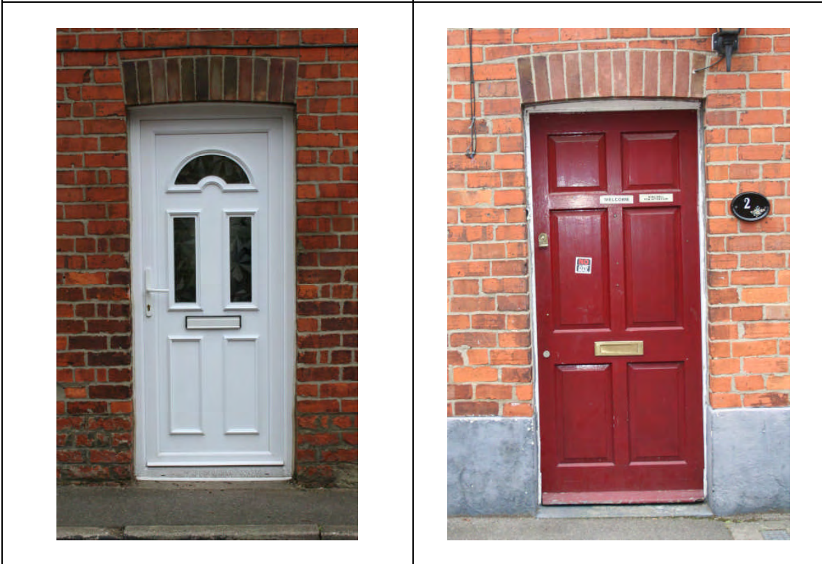
Plate 41: These doors and windows are from a matched pair of houses. The one to the left has lost its character through the use of UPVC, the one to the right retains its painted timber details.
