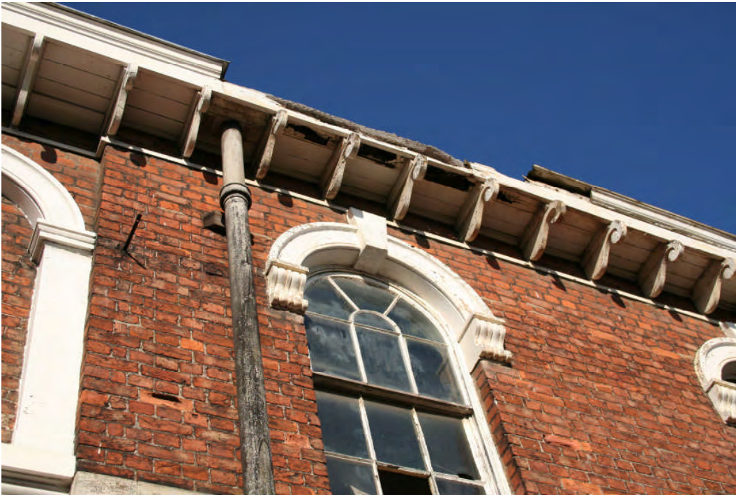
Plate 64: One of the many failures on this listed property on High Street
