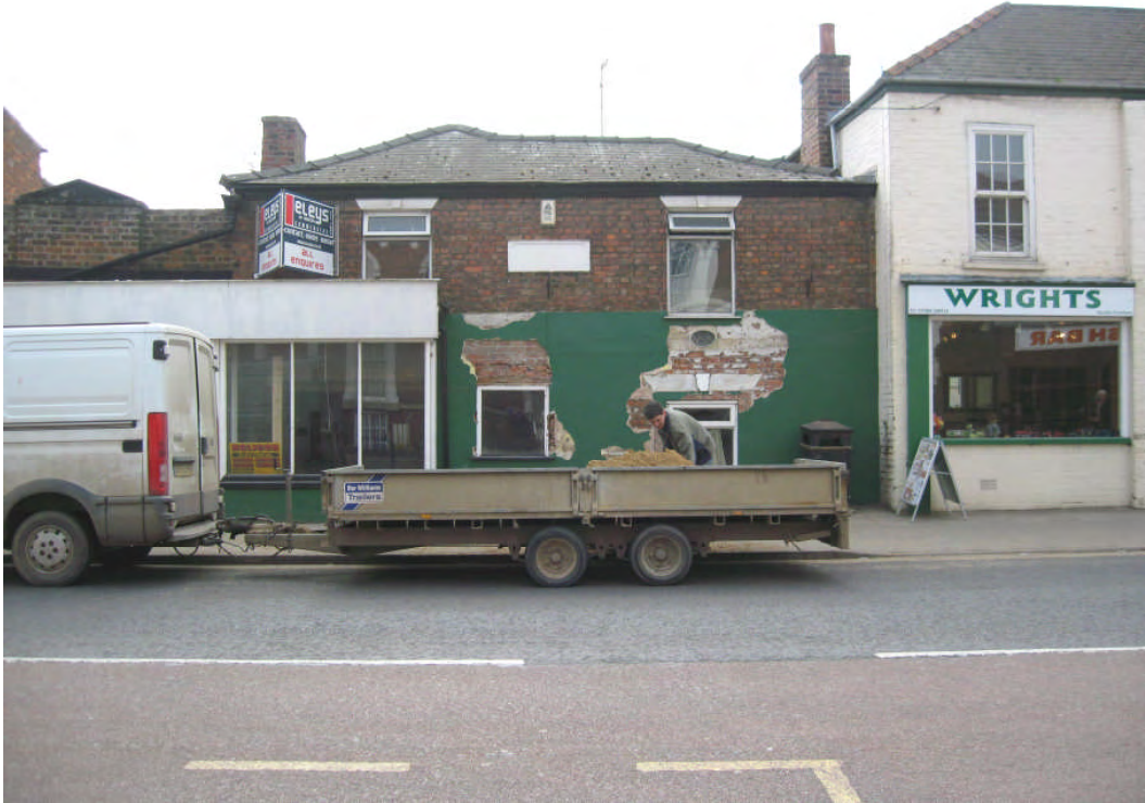
Plate 66: A property in poor condition which is benefiting from the current grant scheme
