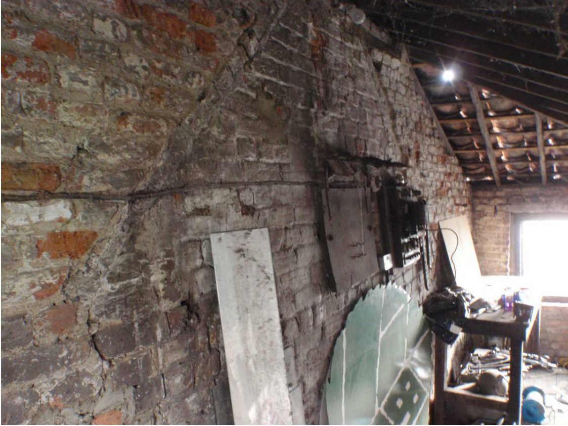
Plate 9 Two-storey southern block, upper floor, showing lines of original gable, looking northwest
