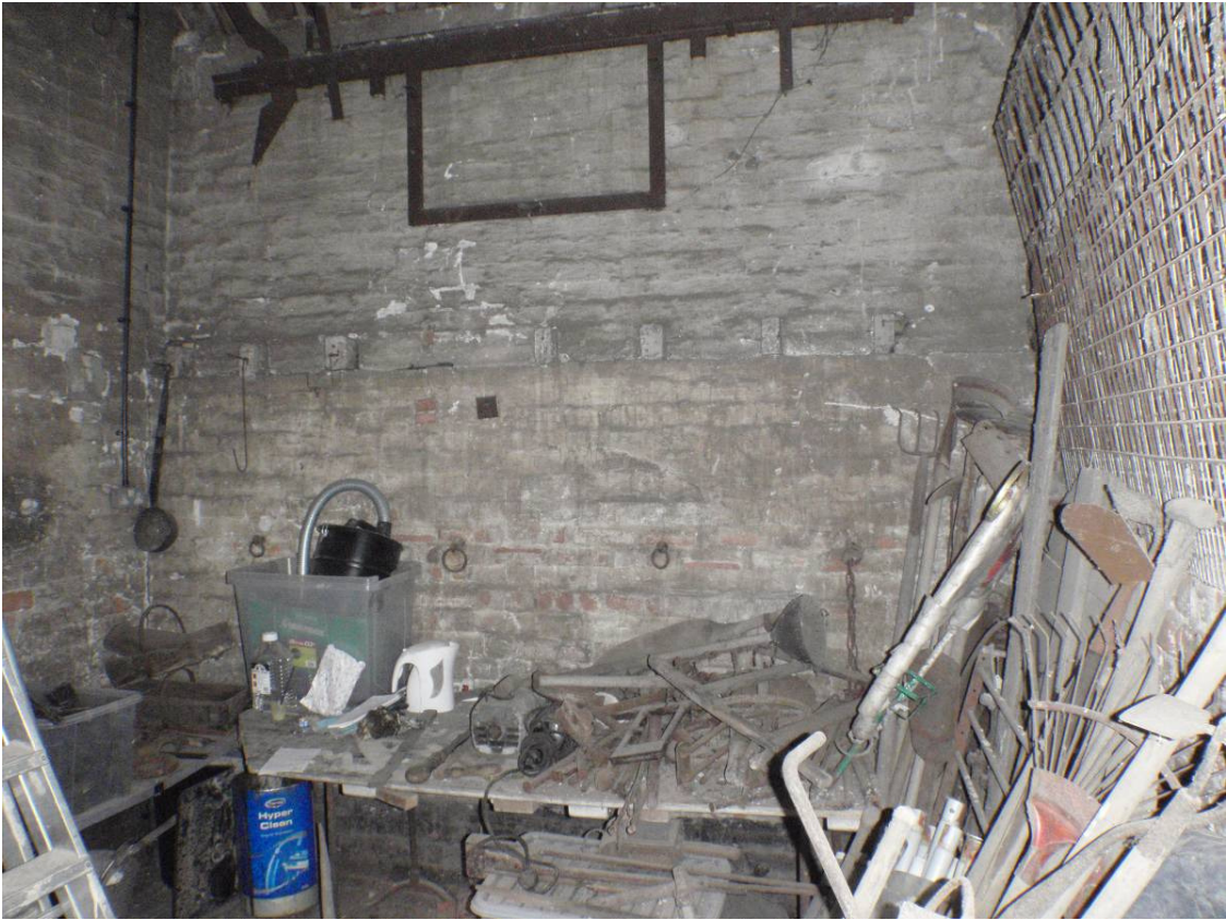
Plate 21 West wall of northern room, showing line of tether rings, looking west
